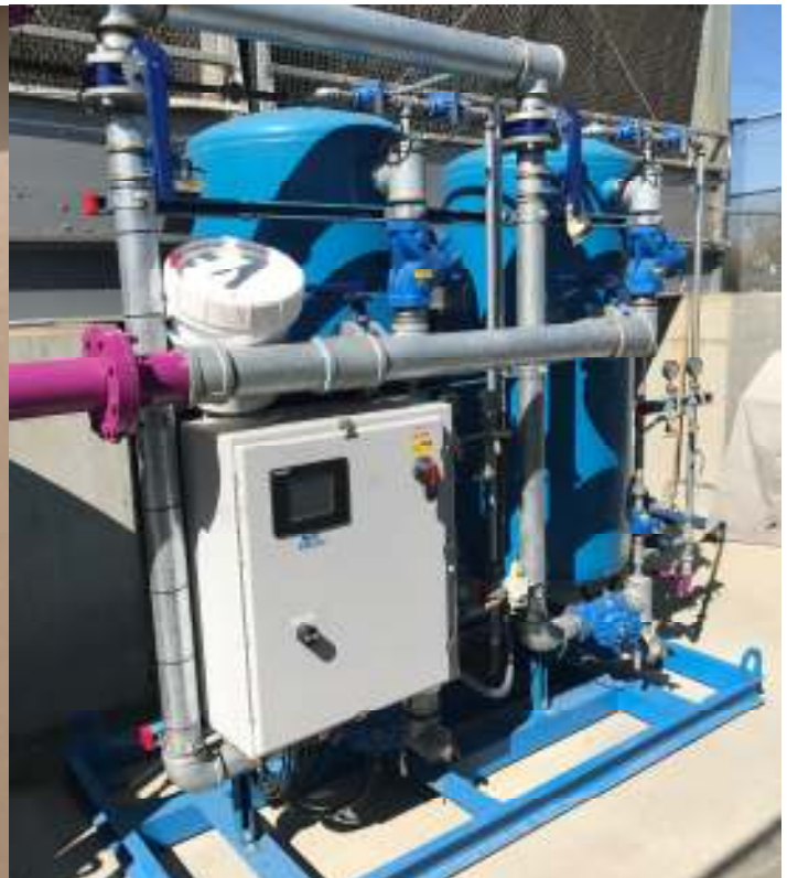
Water Treatment/Softener System
